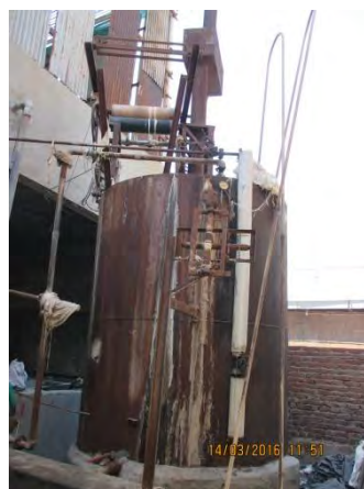
Caption: Kier Boiler at Rajkumar Textile
