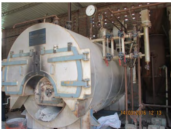
Caption: Boiler unit at Rajkumar Textile
